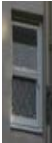
Timber frame. Timber sashes Double hung. Diamond leadlight to bottom sash. Obscure glass to top sash.
